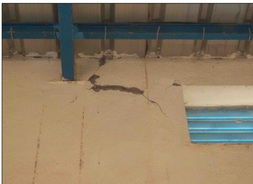
Cracks found largely in the interior walls of schools (Kanembakache school, Department of Mayahi, Maradi Region)
