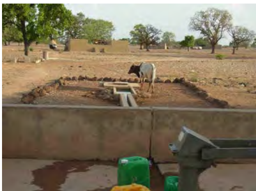
Spilled water from the pump flows to livestock watering hole through drainage
