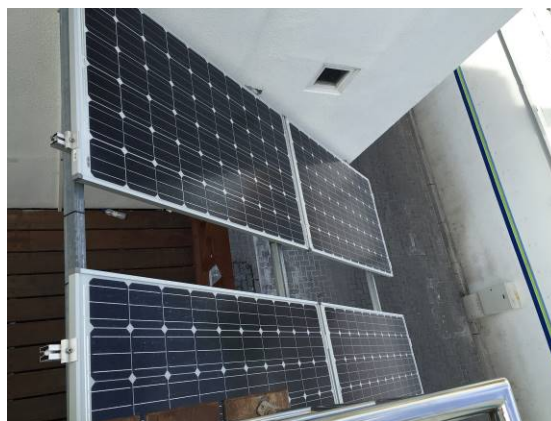
MEE's Self-Financed Solar Panels (Building of MEE)
