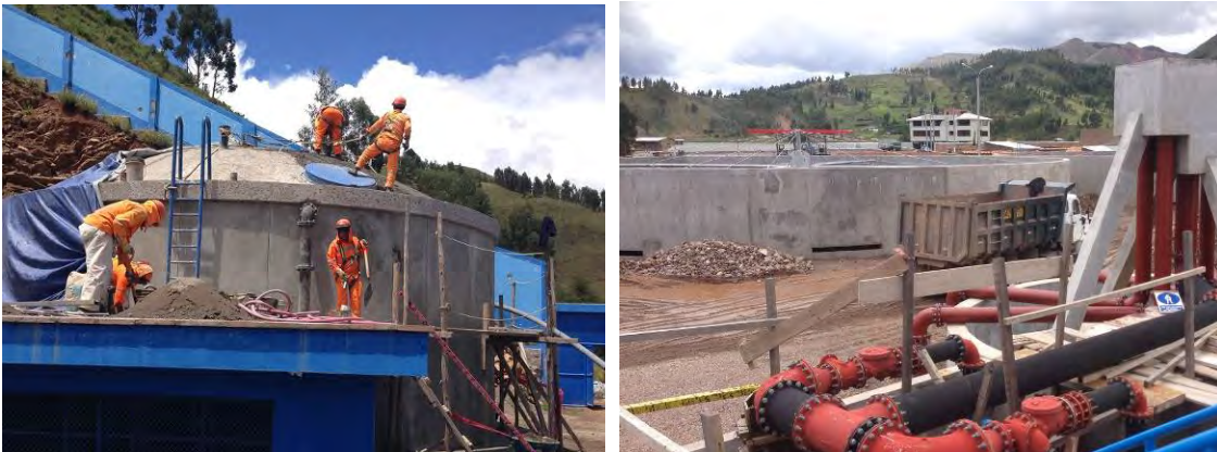
Water distribution reservoir (left) and waste water treatment plant (right) under construction in Sicuani
