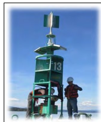
Routine maintenance of buoy (provided by CEPA)
