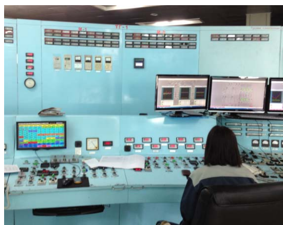
Fig.4.2-20 Turbine Control Panel in CCR
