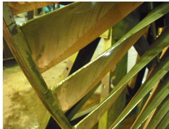
Fig.4.2-17 LP Last Blade after Repair
