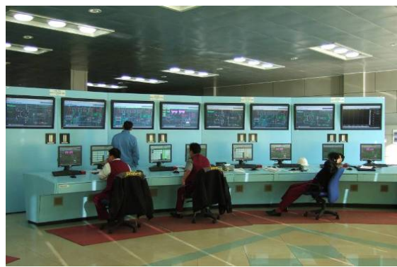
Fig.4.2-19 Boiler Control System after Modification
