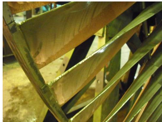
Fig.4.2-17 LP Last Blade after Repair
