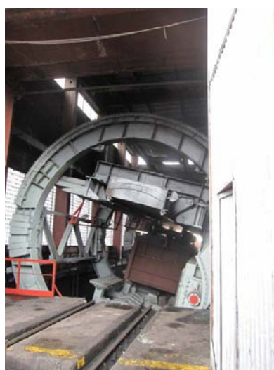
Fig.4.2-29 Coal Unloading Facility of TPP4
