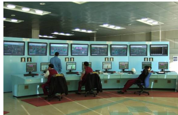
Fig.4.2-19 Boiler Control System after Modification
