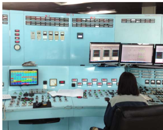
Fig.4.2-20 Turbine Control Panel in CCR
