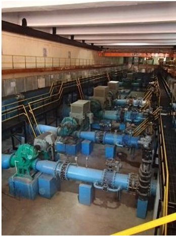
Jawahar circle pumping station
