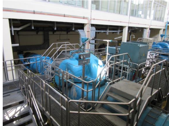
Pump installed in this project (Phet Kasem Distribution Pumping Station)
