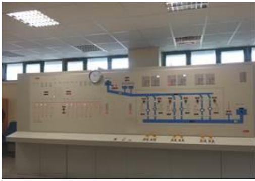
Control Room in the Treatment Plant
