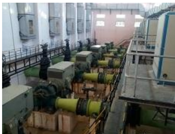
Balawala pumping station
