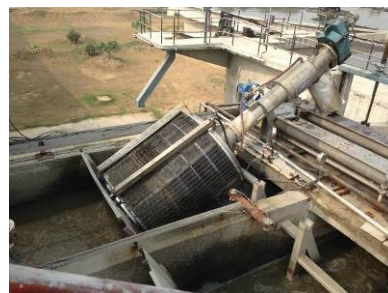
Sewerage Treatment Plant (Keshopur)
