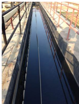
Sewerage Treatment Plant (Western area)
