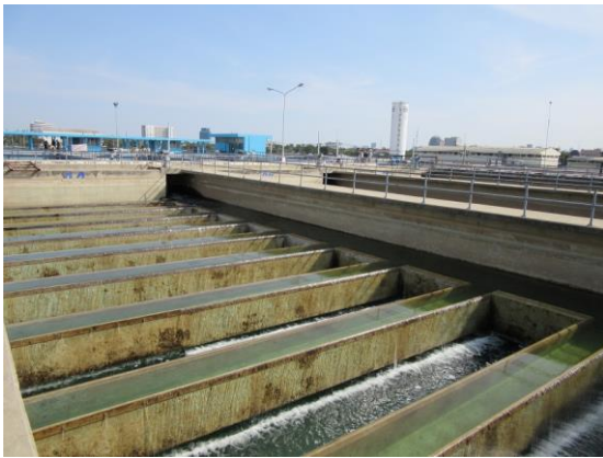
Bang Khen Water Treatment Plant (section expanded in this project)
