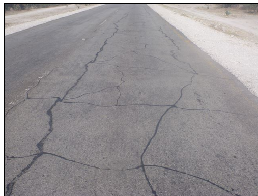
Surface cracks (after repair works, near Bunya)
