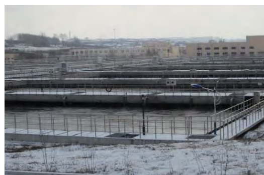
A reaction tank at the Pingfang sewage treatment plant
