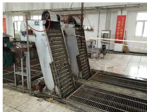
Coarse screens at a sewage treatment plant
