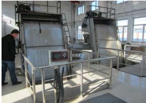
Inlet filter of the Zhanggaiying
