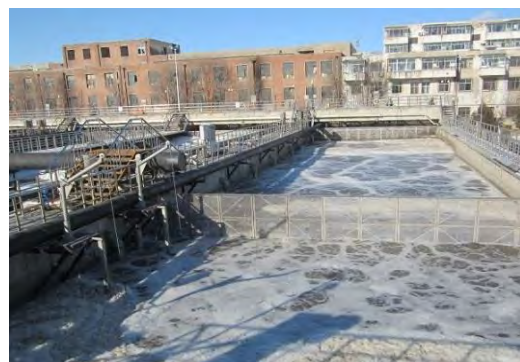
Bio-reaction tank in the Gongzhufu sewage treatment plant
