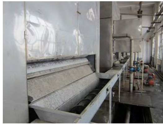
Sludge treatment facilities at the Pingfang sewage treatment plant
