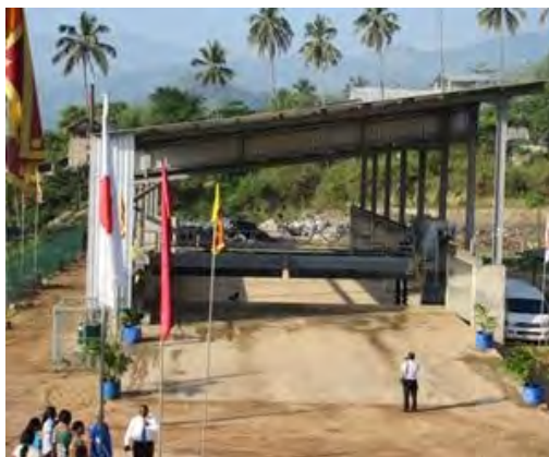
Overall view of the composting plant
