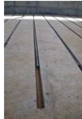
Channels in the floor and aeration pipes
