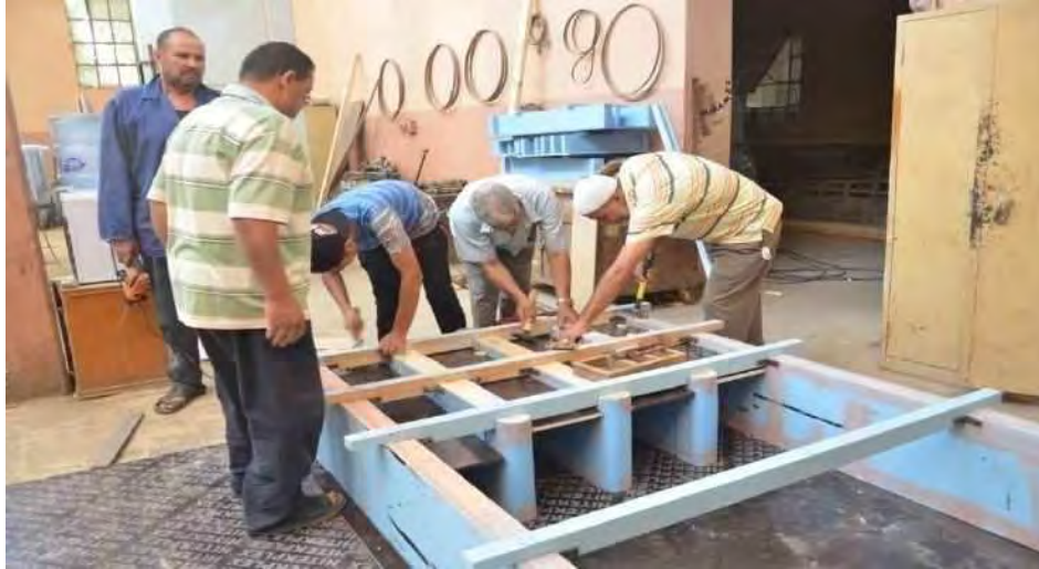
Figure 5: Manufacturing of the New Regulators in the HRI workshop
