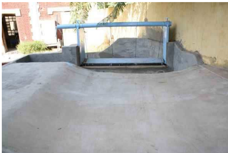
Photo (9): Mounted End Tail Gate for El-Ibrahimia Canal
