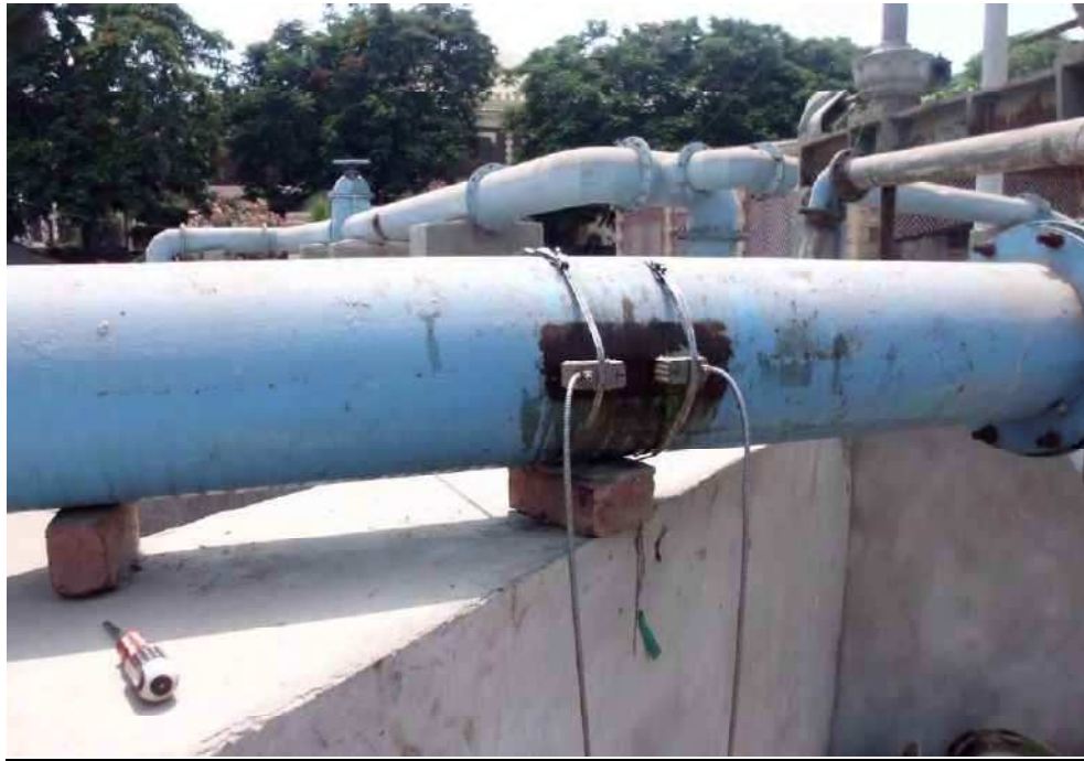
Photo (4): Fixed Ultrasonic Flow Meter around Feeding Pipe
