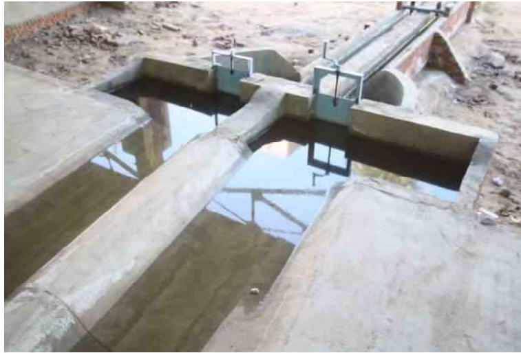
Photo (6): End Tail Gate of Badraman and Daytutiah Canals
