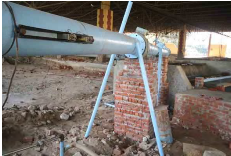
Photo (22): Fixed Ultrasonic Flow Meter around Feeding Pipe
