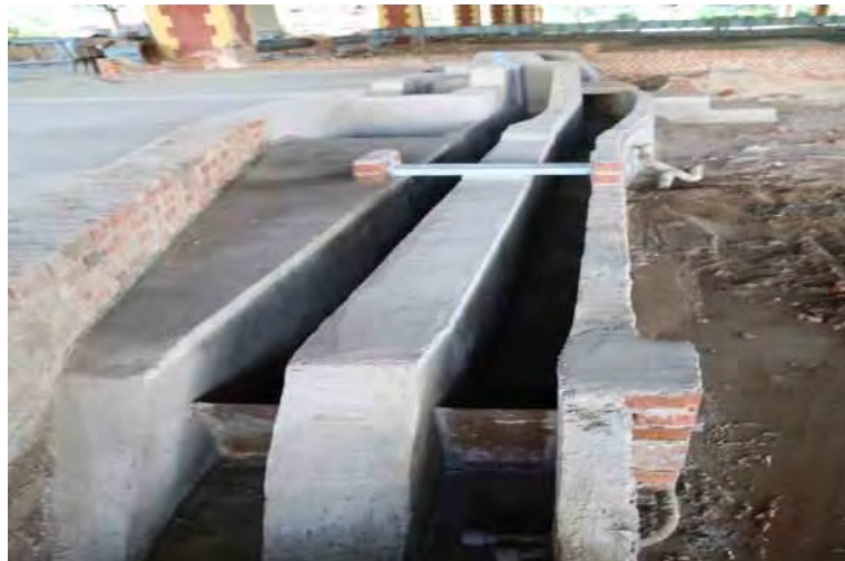
Photo (5): Sharp Crested Weirs for Irad Delgaw and Abou Gabal Canals
