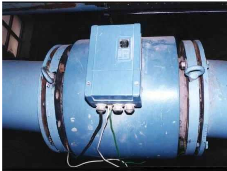
Photo (21): The Electro-Magnetic Flow-Meter
