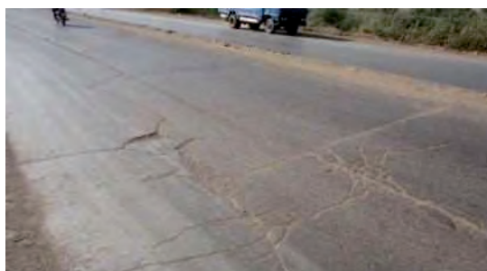
Photo Pavement damage example (cracking at sag section)
