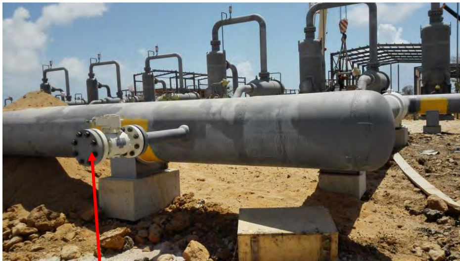
Typical tapping point at SomangaFungu. This point will supply natural gas to Kilwa Energy power plant and any other,
