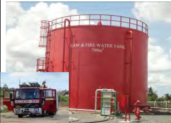
Raw & Fire Water Tank (+Fire engine)
