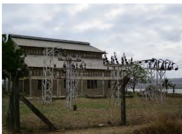
Former / Old DG Plant
