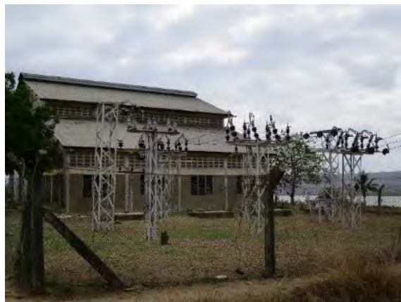
Former / Old DG Plant
