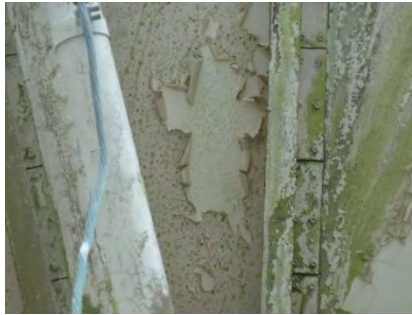
Picture 11: Peeling Paint on Rear of Main Reflector
