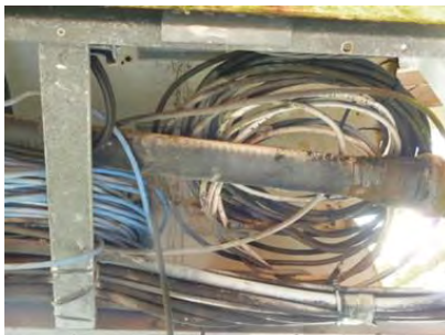
Picture 15: Significant Deterioration of Cable and Waveguide outer jackets
