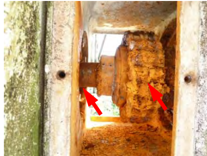
Picture 5: EL (elevation) Motor Shaft
