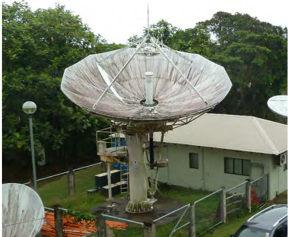
USPNet C Band Parabolic Antenna Photographer: Project worker (November 2015)
