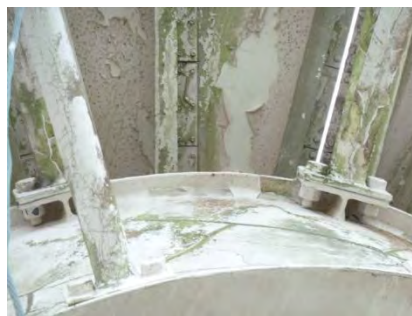
Picture 12: Peeling Paint on Rear of Main Reflector/Outer Surface of Center Hub
