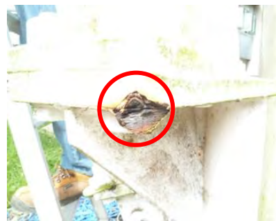
Picture 10: Rust Causing Pedestal Curling
