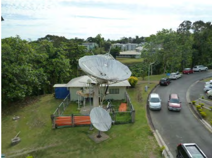
USPNet Satellite Earth Station Photographer: Project worker (November 2015)
