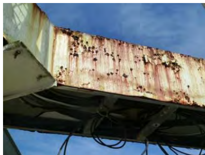
Picture 14: Deterioration of Cable Ladder Housing Due to Rust
