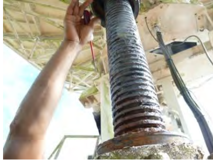
Picture 8: EL Jack Shaft
