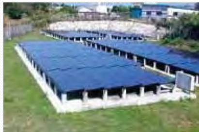
Survey, planning, and construction work management of 200 kW PV project in Kita Daito Island
