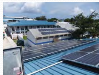
Preparatory study for sustainable system development project for remote islands (operation of diesel generators) (JICA project)
