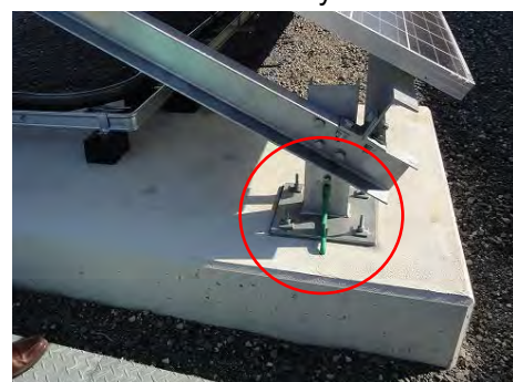
Earth wire connected to a rack
