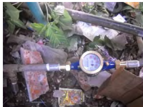
Photo 4.11 High Position of Water Meter
