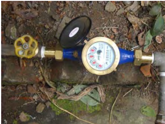
Photo 4.1 Installed water meter
