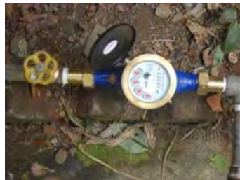
Installed water meter
