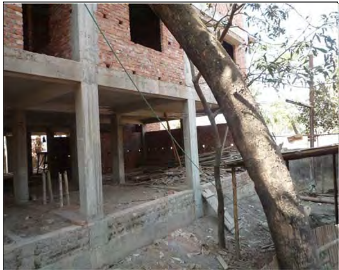
The building under construction by CWASA in Halishahar. Meter testing will be set on the ground floor.
