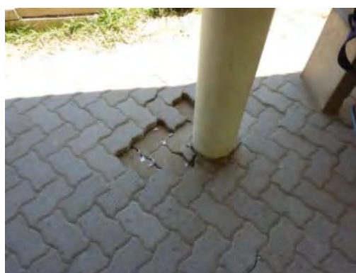
Photo 12: Subsided blocks (Nkobe school)
