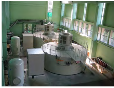
Generator (Unit 1, Unit 2)
