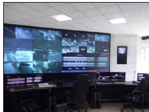
Photo 5: Control Centre of Tunnel
