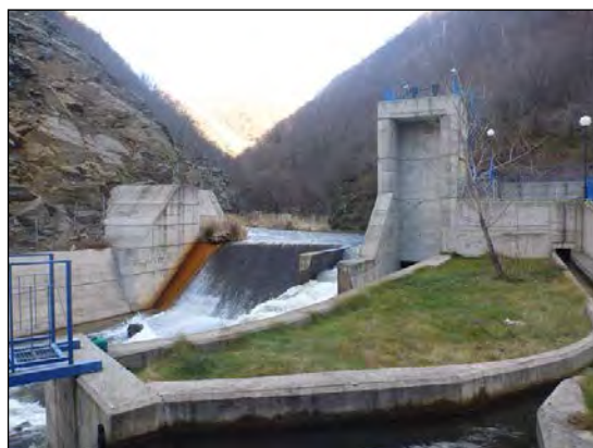
Photo 1: Water Intake No.1
