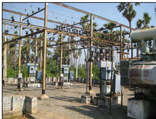
A substation constructed by the project (Andhra Pradesh State)
