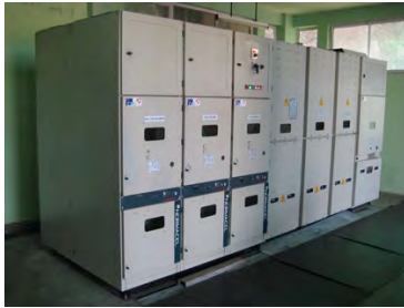
11KV Switch Gear Panel
