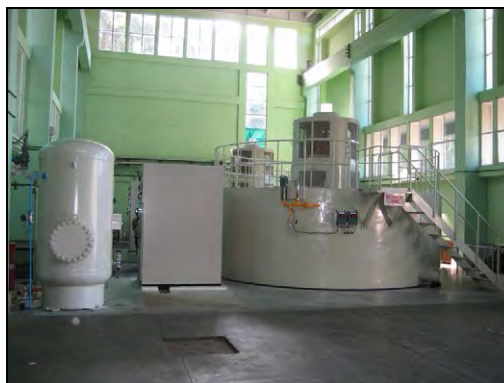
The Generator of the Uiam Stage II Hydro Power Station
