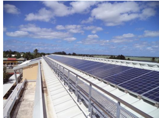
Solar panels installed in this project
