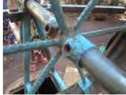
Photo. 5. The wheel of a rope pump that is not working because it has had its bolt removed (Bolosore Woreda, Wolayita Zone) (Photo by the evaluator)
