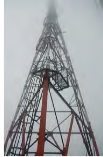
Antenna Tower at Grand Etang (at the time of the Ex-Post Evaluation)
