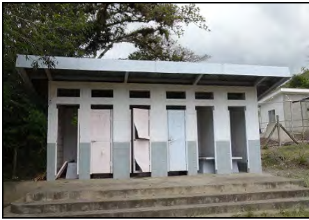
External view of pit latrines (six booths. Doors have come off in three of them and cannot be used)
