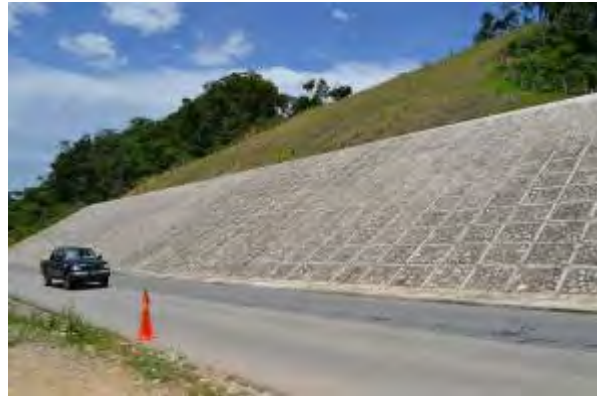
Slope Protection Works on National Road 1 in Variante, Tarija Department (Pilot Project)
