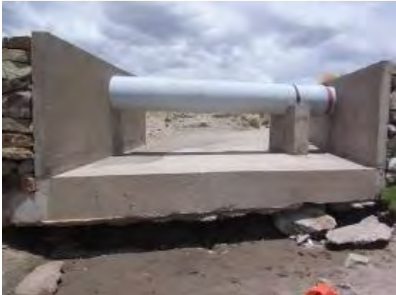
Scouring of foundations around the protection work of the conduction
