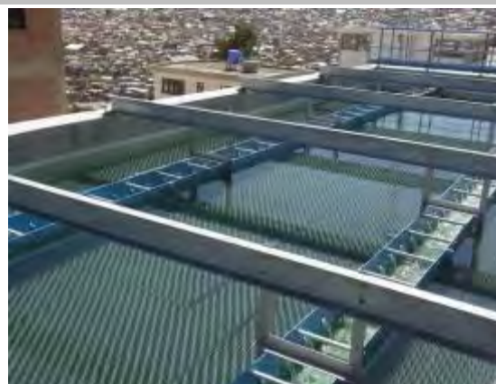
Rio San Juan Water Treatment Plant
