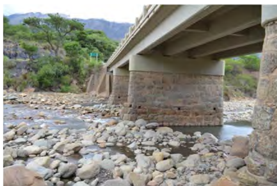
Repair of Popo Bridge on National Road 7 Cracks in the main girders and floor plates were repaired, giving the bridge the strength to withstand the weight of large vehicles. (Pilot project)
