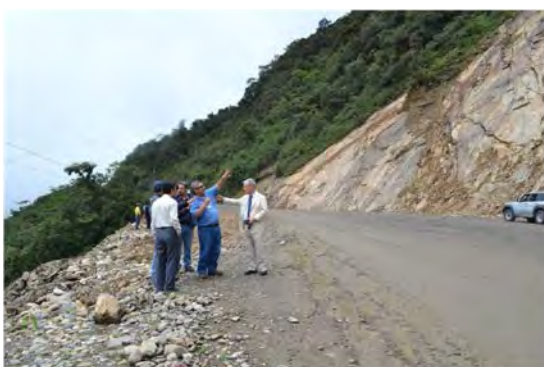
Site of slope failure on National Road 4 Due to the extensive slope failure, the road width is much larger than usual.
