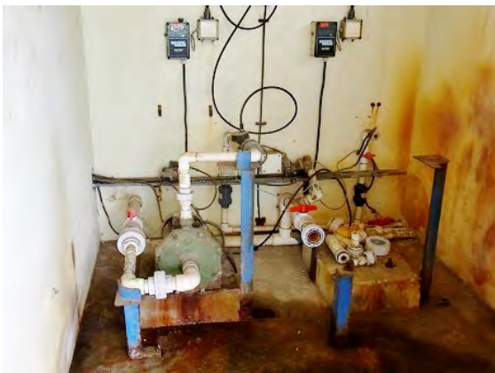
A well for which one of the chlorine injection pumps was removed to take spare parts (Friendship Well)
