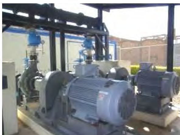
Siglo XX Pumping Station
