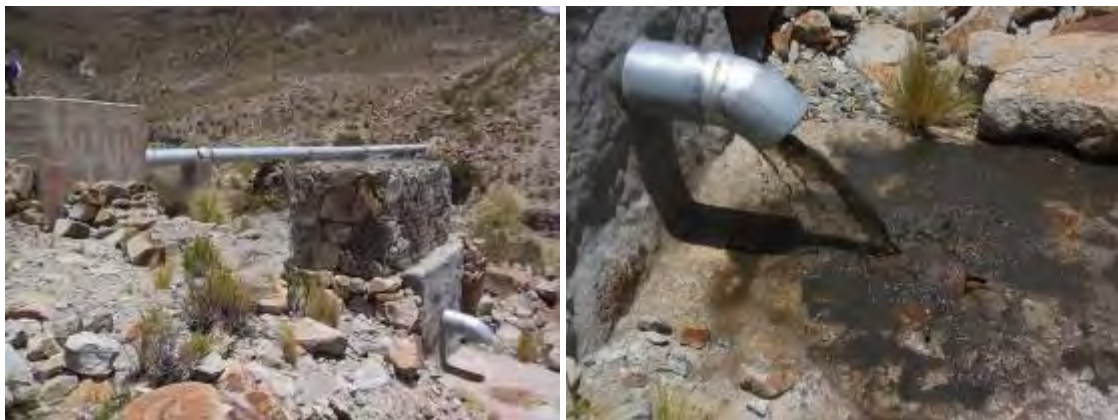
The dirt removal facility
