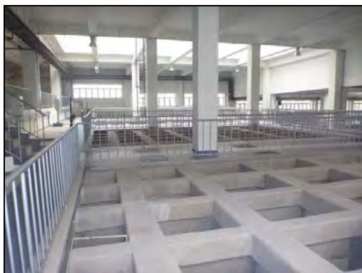
Photo 1: Inside of Water Treatment Plant
