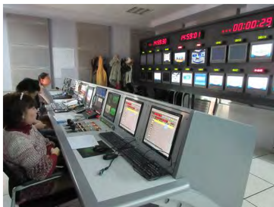
Studio monitor room during on-air operations, JLTV
