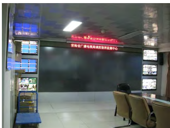
Broadcast Control and Monitoring Center (Qinghai Radio Film and Television Bureau)
