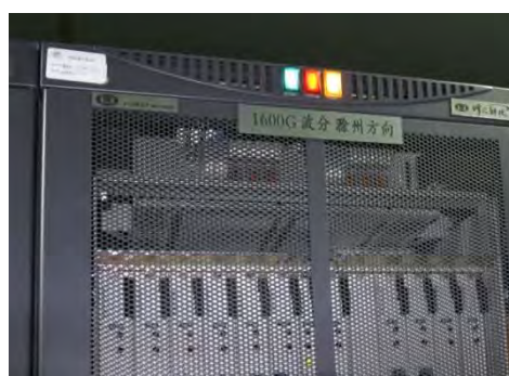
Equipment of cable network in ARTTC
