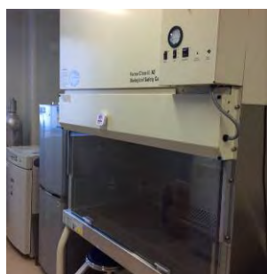
A biological safety cabinet installed at a prefectural CDC (Xinxiang).
