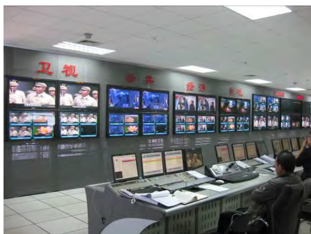
TV Control Room
