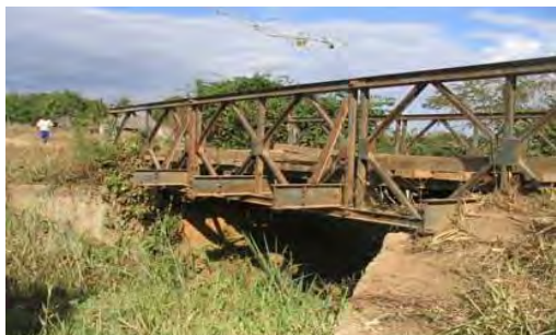
(Source) Preparatory Survey Report Figure 3: Bridge Subject to Flooding Before the Project
