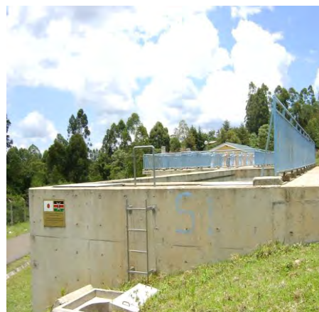
Sedimentation Pond of the Water Treatment Plant
