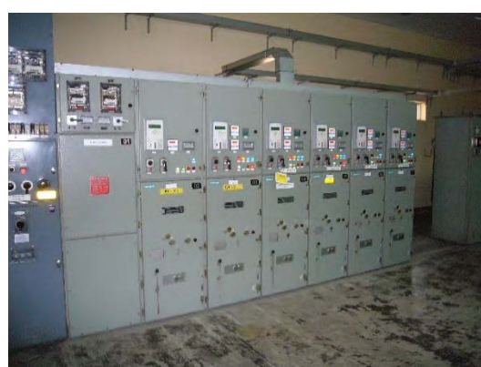
Primary Substation “H” (Inside)
