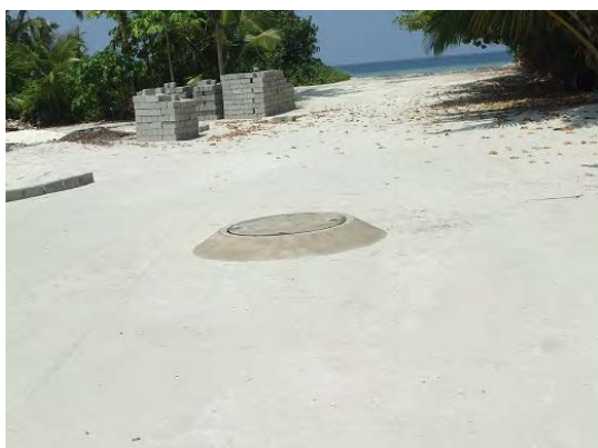
Sewerage pumping station, Funadhoo
