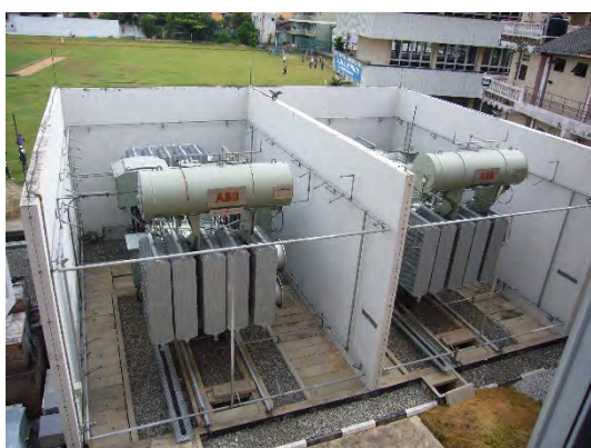
Primary Substation “H” (Outside)
