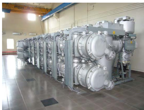
Kelanitissa Substation (inside)
