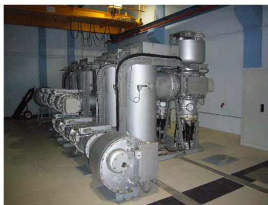
Inside of Substation “C”
