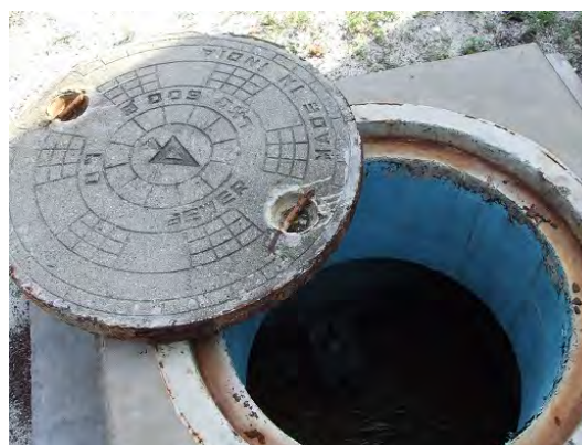
Sewerage pumping station, Eydhafushi
