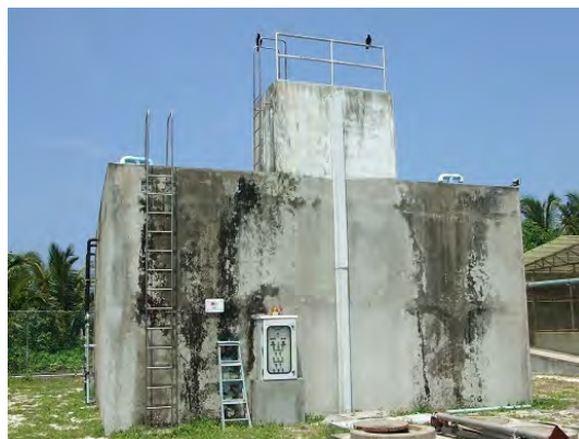
Muli wastewater treatment plant
