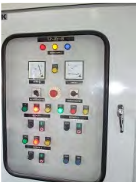
Control panel of wastewater treatment plant, Fenaka (Eydhafushi)
