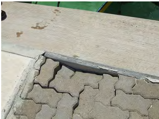
Fonadhoo harbour: dent on quay wall (other harbours have similar dents)
