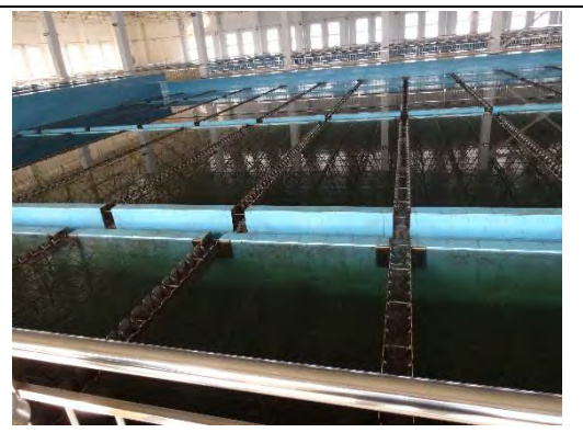
Photo 3: The 150,000 m 3 /day Purification Plant Constructed in the Sub-project
