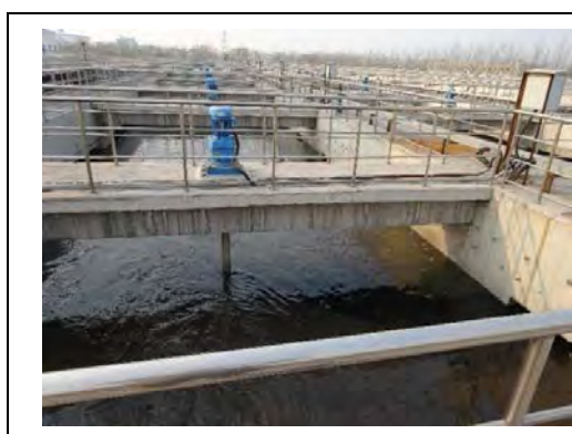
Photo 4: A Primary Sedimentation Pond in Dadaowan Wastewater Treatment Plant 19
