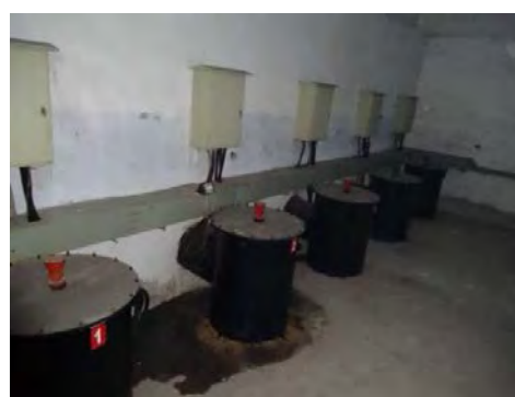
Photo 5: The Wastewater Pumps Additionally Adopted in the Sub-project
