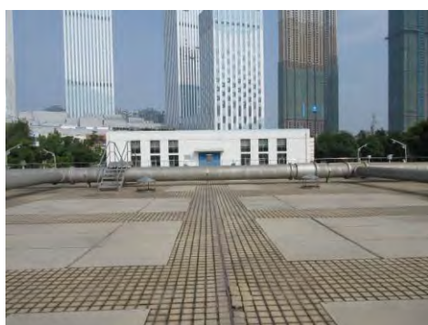
Photo 4: The biological reaction pool of the Treatment Plant
