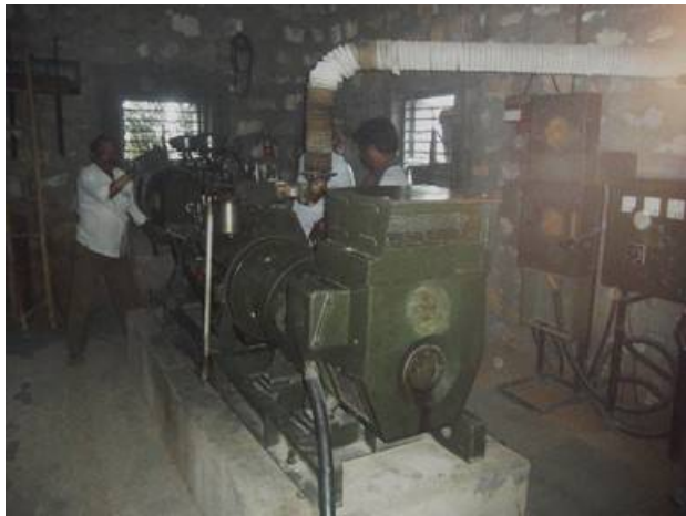
(Generator House) Generator: Replacement
