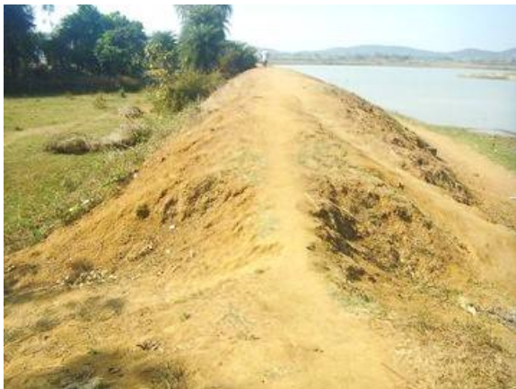
Tank bund is seriously damaged, which shall be improved along with intake structures, spillway and canals. (Vizianagaram District)
