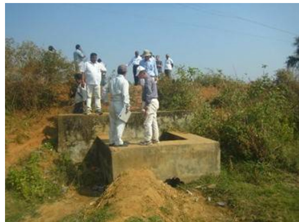
The earth canal is not functioned due to sandy soils, which requires concrete lining. (Vizianagaram District)
