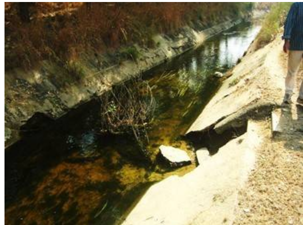
Concrete lining of main canal shall be partially repaired due to damage. (Chittoor District)
