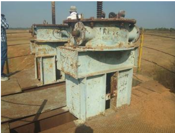
Malfunctioned old intake gates shall be replaced with new ones. (West Godavari District)
