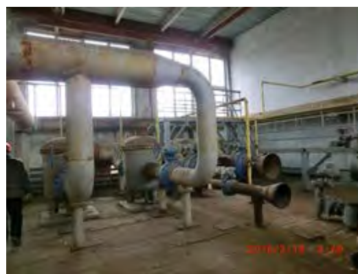
(Gas receiving facility)
