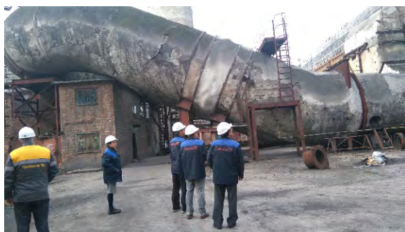
(Flue Gas Duct between boiler and chimney)
