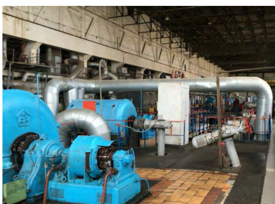
(No.1/2 Steam Turbine)
