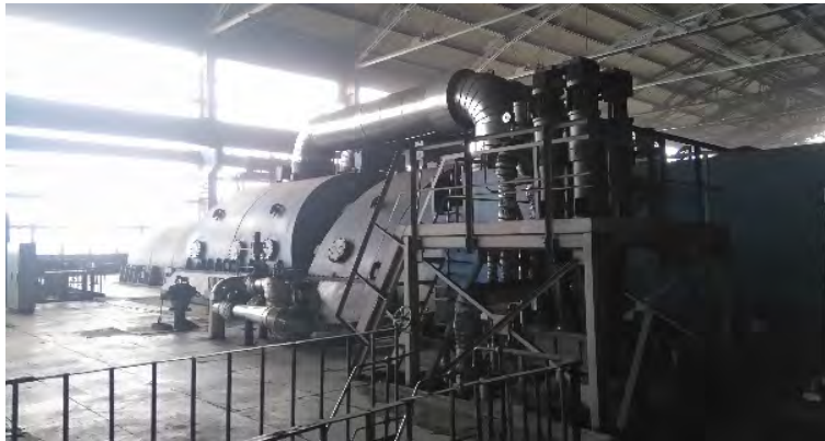
Figure 5.2-2 No.4 Steam Turbine
