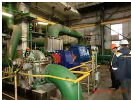
(Hot water supply pump)
