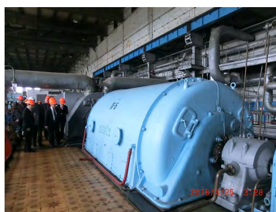
(No.4 Steam Turbine)
