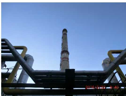
(Exterior of CHP-2)
