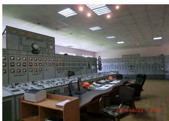
(Central Control Room)
