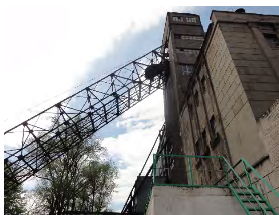
(Coal Handling Conveyor)
