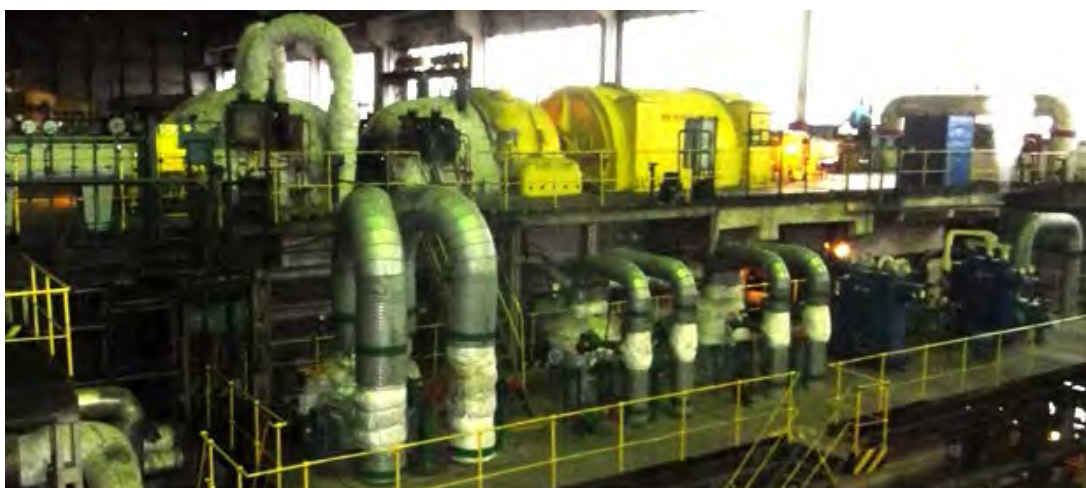
(No.2 steam turbine (PT-50-130 by Skoda, from left to right, high pressure and intermediate-low pressure turbines, and generator))
