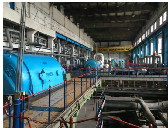
(Siemens-make Steam Turbine)
