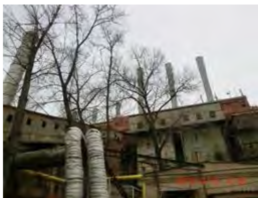
Figure 7.3-1 Exterior of Kyivenergo CT-1
