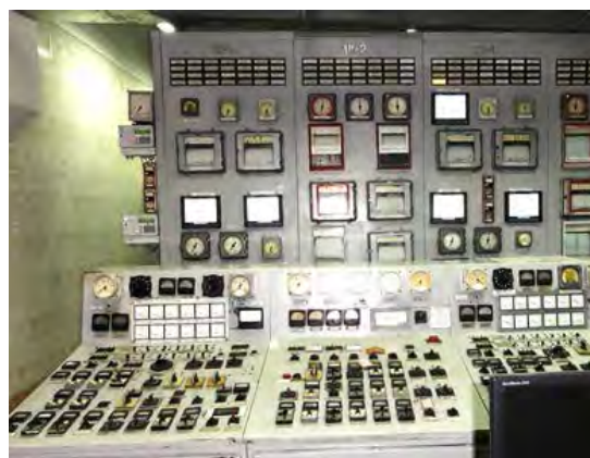
(Boiler control panel (partially updated to digital representation))
