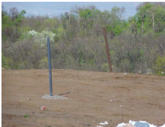
(Collecting pipes of generated methane)
