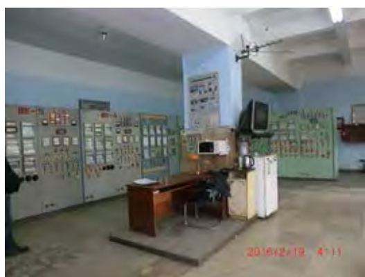
(Central control room)
