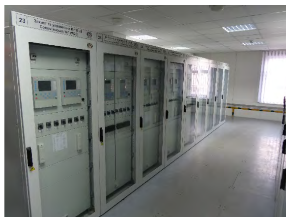
Figure 6.4-2 Digital Protection Relay Panel
