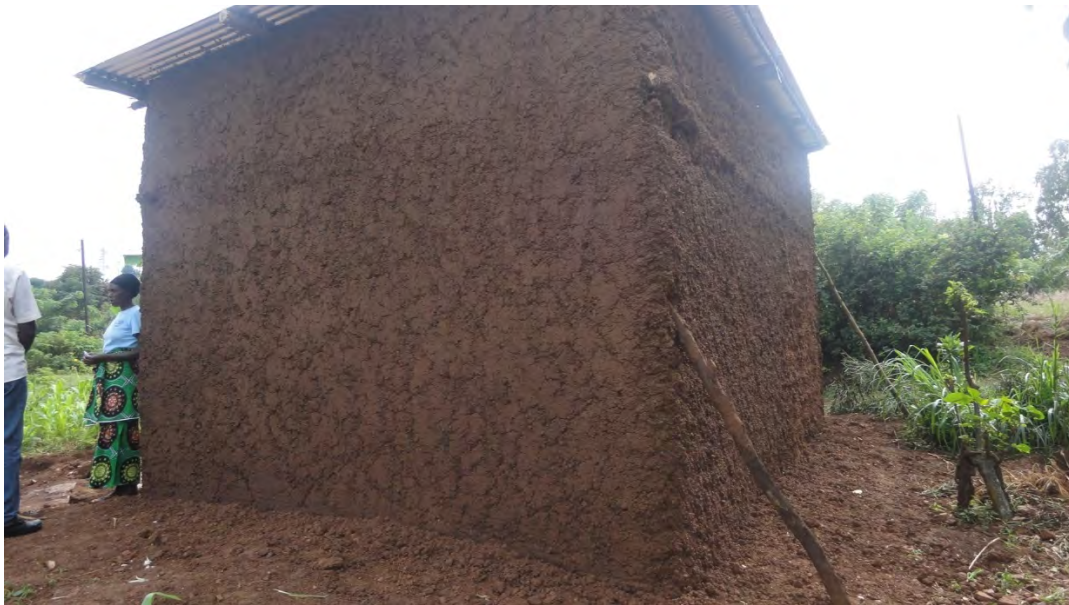
Figure 5: Building in Ndera Sector affected by the project
