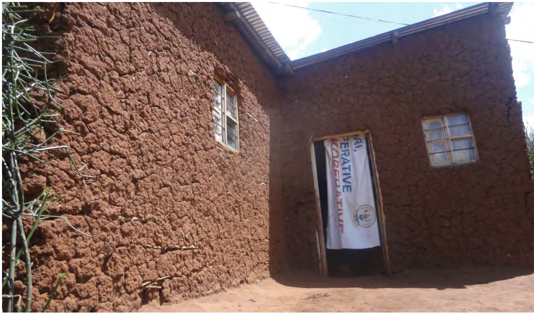
Figure 4: Second building in Bumbogo Sector affected.
