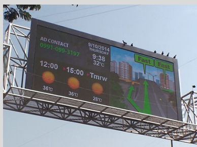
Traffic boards installed in four city-locations for this operation (Photo: Zero-Sum Ltd.)
