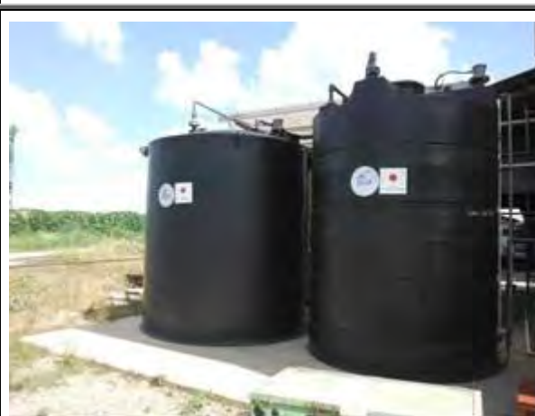
Rainwater recovery system
