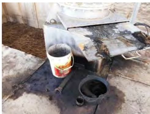
Leakage of Wood Vinegar from the Damper
