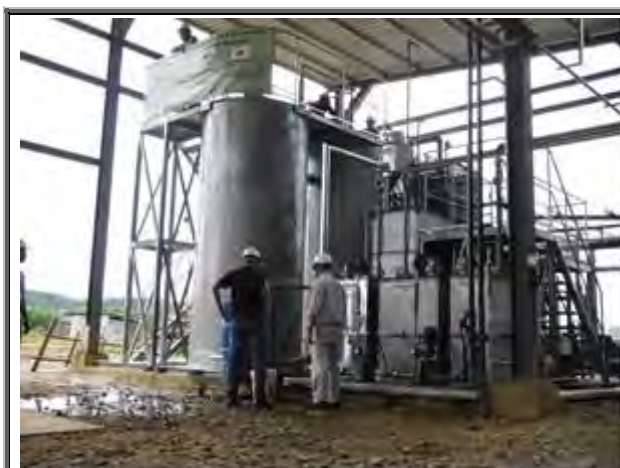
Anaerobic and Aerobic Bioreactors
