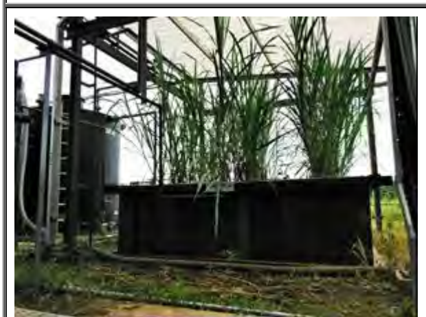
Final effluent polishing system by Engineered Wetland
