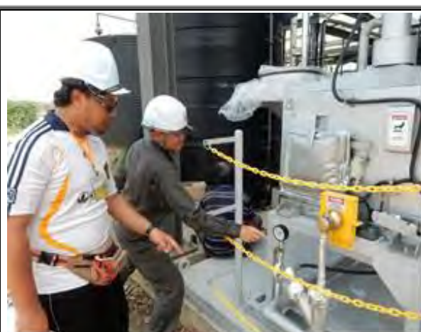
Energy and water recovery system from waste steam
