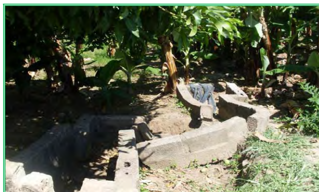
Figure Irrigation infrastructure destroyed by hippos and elephants at Kapululira Banana Irrigation Scheme (Siavonga District).
