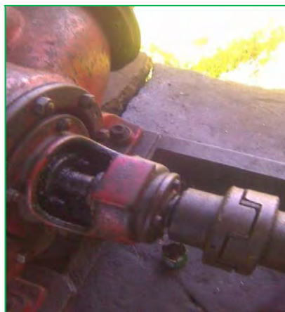
Figure Spilled used oil at Kapululira Scheme pump
