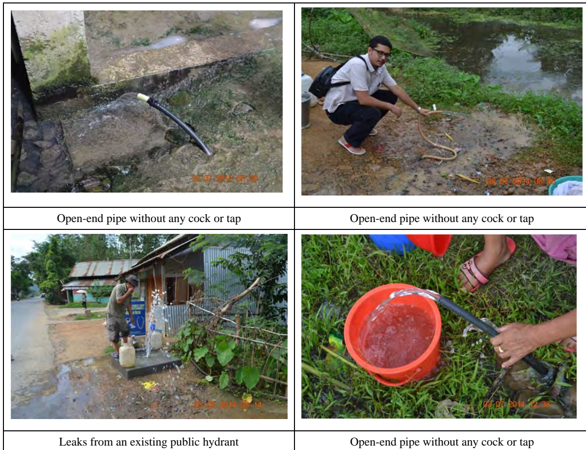
Photo 6.1 Conditions of Existing Faucets
