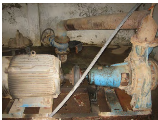
Photo 2.10 Clear Water Pump at Porompat-I (for Porompat Zone)
