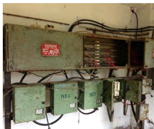
Photo 2.5 Incoming and distribution panels at Singda WTP
