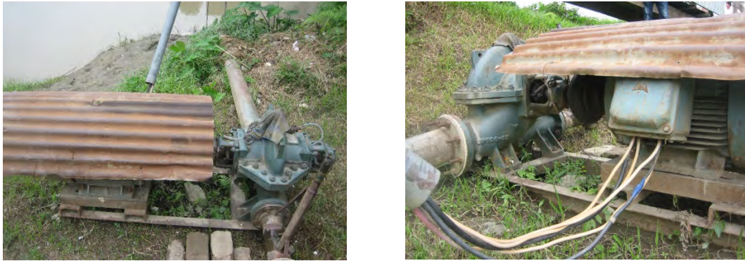
Photo 2.2 Raw Water Pump at Ningthempukhri Intake Work
