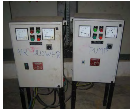
Photo 2.9 Starter panels for air blower and backwash pump at Kangchup WTP
