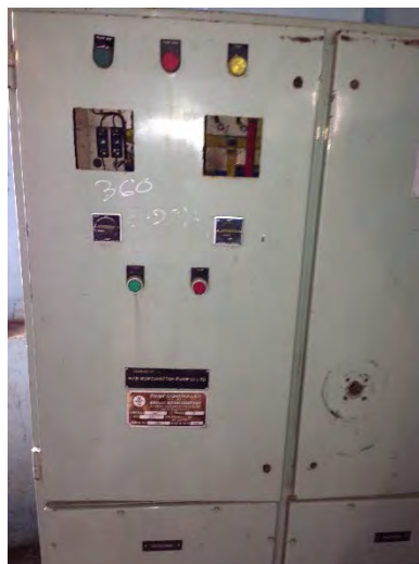
Photo 2.3 Raw Water Pump Starter Panels at Porompat Intake Works
