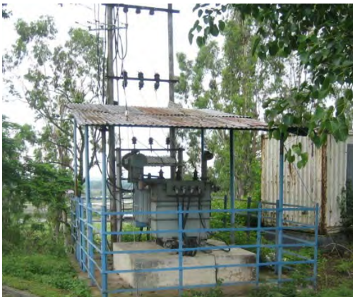
Photo 2.8 Transformer at Kangchup WTP
