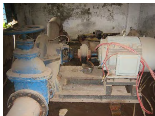
Photo 2.11 Clear Water Pump at Porompat-I (for OHT)
