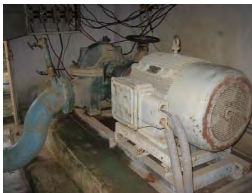
Photo 2.12 Clear Water Pump at Old Thumbuthong WTP
