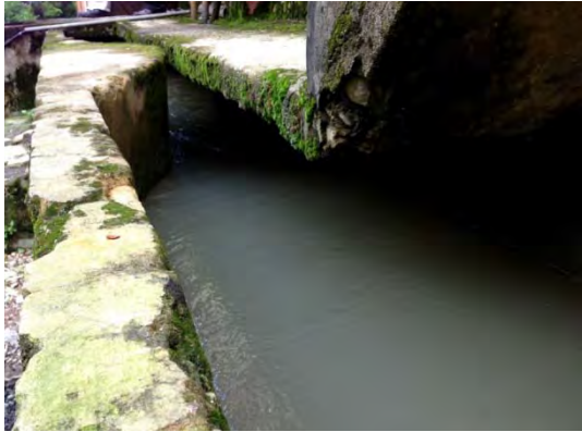
Photo 2.6 Parshall flume at Singda WTP
