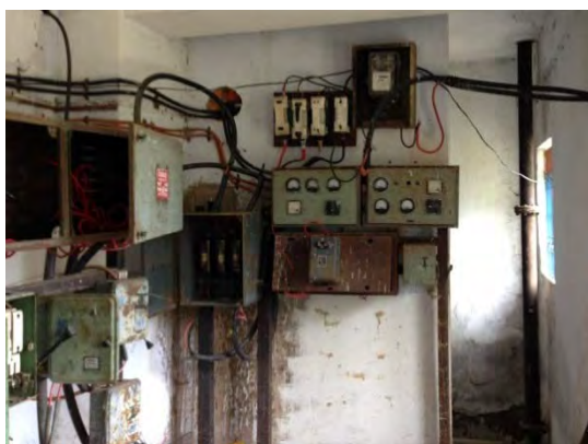
Photo 2.4 Watt-hour meter at Singda WTP
