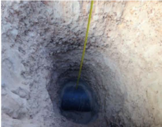
Test Pit No.15 (300DIP Pipe Found) Over 2m-Dept)
