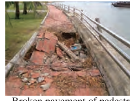
Broken pavement of pedestrian walkway (Bai Chay)
