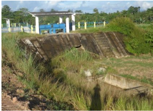
Note: Damaged by Flood. Photo taken in May 2014
