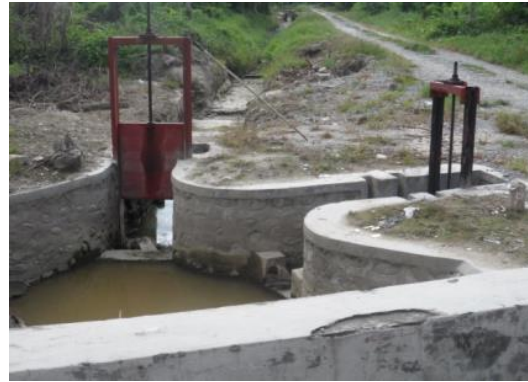
Note: Mud pile is hindering water distribution. Photo taken in May 2014
