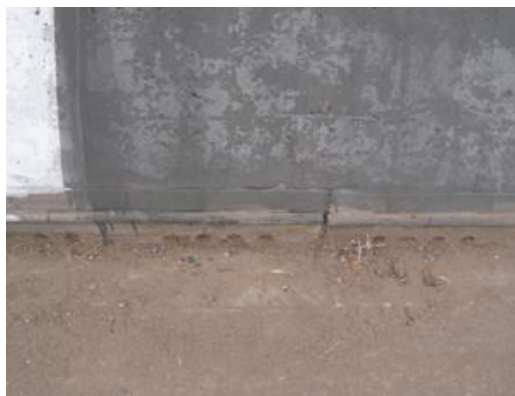
Photo5. Road side of Balaraja FO (sand still remains inside the drainage system after cleaning)
