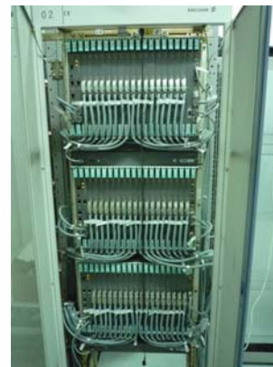
Digital Switching System
