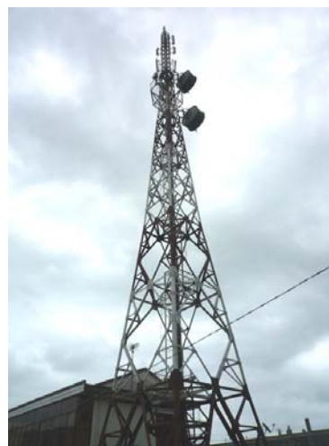
Microwave Transmission Tower
