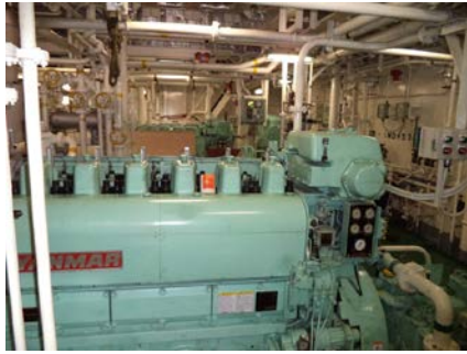
Photo 3: Engine Room maintained in clean condition
