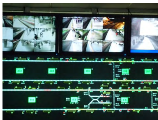
Remote Control and Surveillance System
