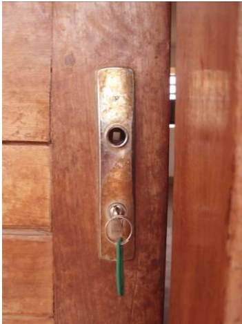
Figure 4. Vulnerable Door Handle
