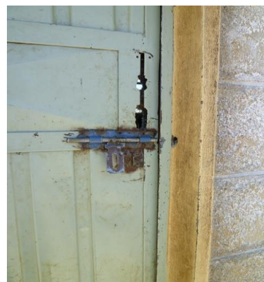
Figure 2 Broken door knob & key hole that is changed to a bar key
