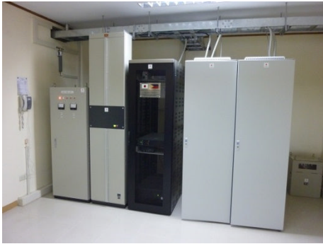
Photo 5: Data Processing System inside Agno Sub Center
