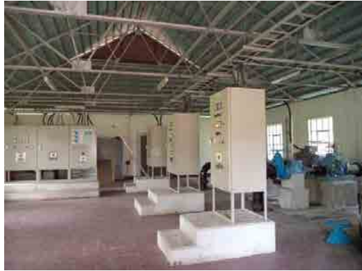
Photo 1: Saateni Station Transmission Pump House
