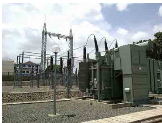
Makumbusho Substation developed in this project
