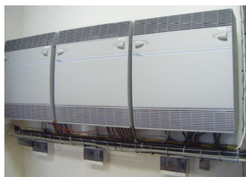
Installed communication equipment
