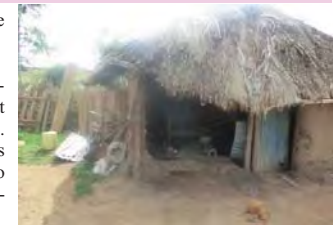
Aftermath of floods: Damaged houses that are yet to be reconstructed
