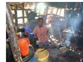
Child standing inside their house that has been affected by flooding. Notice the wet floor and the broken walls
