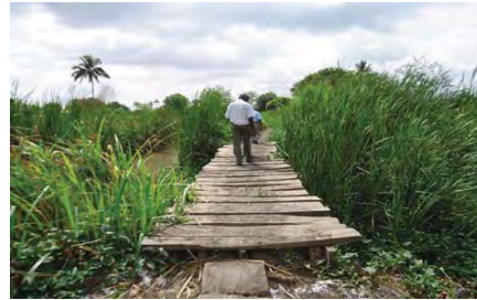
Wooden Footbridge constructed by the community to assist in crossing of Lumi for the 2 villages of Marodo and Majengo
