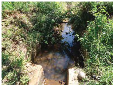
Silt Trap to prevent excessive deposition in reservoir
