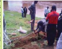
WRUA members dig trench to lay in cabling pipes that links the gadget at the river and alarm at observer's house
