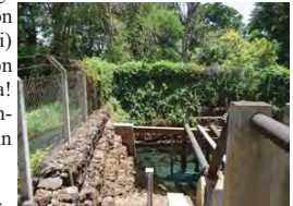
Example of slope protection using Gabions. Situated at the Intake works for Taveta Water Supply adjacent to Njoro Kubwa Springs
