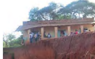
Masaini gully that continuously enlarges due to heavy soil erosion as a result of the flash floods and currently has damaged part of a permanent house structure that is near
