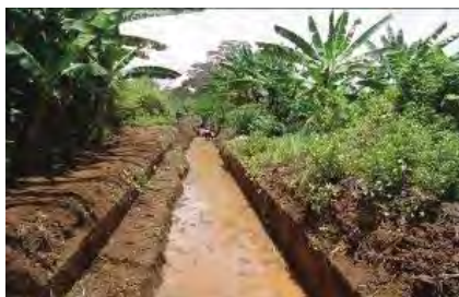
Rehabilitation of Canal in Lower Lumi by WRUA members with funding from WSTF-5 October 2012
