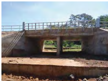
Bridge on River Lumi approximately 2 km from the Kenyan border. All the water has percolated to the ground and then river bed is dry.
