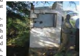
Vandalised Record House
