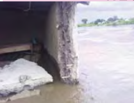
Flood damaged house in Nyora
