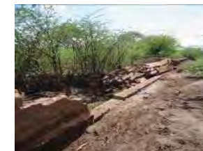
Concrete Wall dyke broken after being hit by flash floods in Laitokok-Taveta Road
