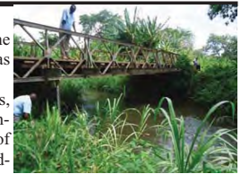
Existing Bridge on River Lumi with a RGS for measuring the water level
