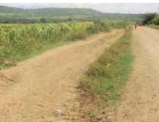
Murrum road which flood water flow on
