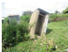
Almost collapsing toilet facility
