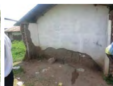
A house seriously damaged by floods
